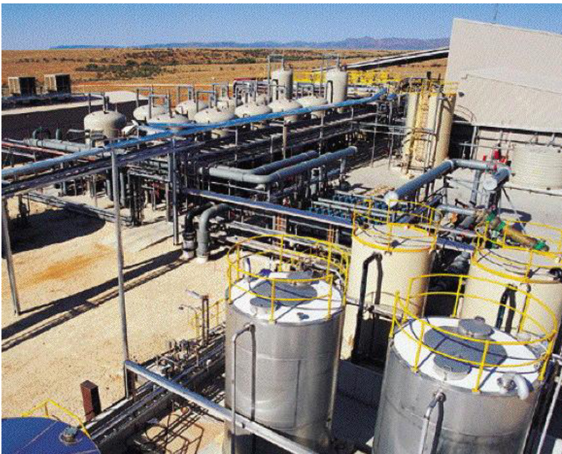
Beverley plant, Heathgate Resources
